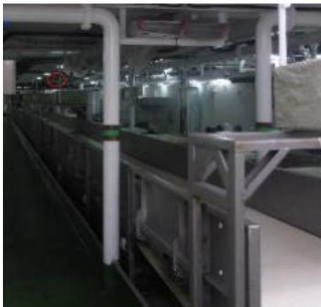
Figure 15: Position of the midships aft viewing conveyor belt camera.
